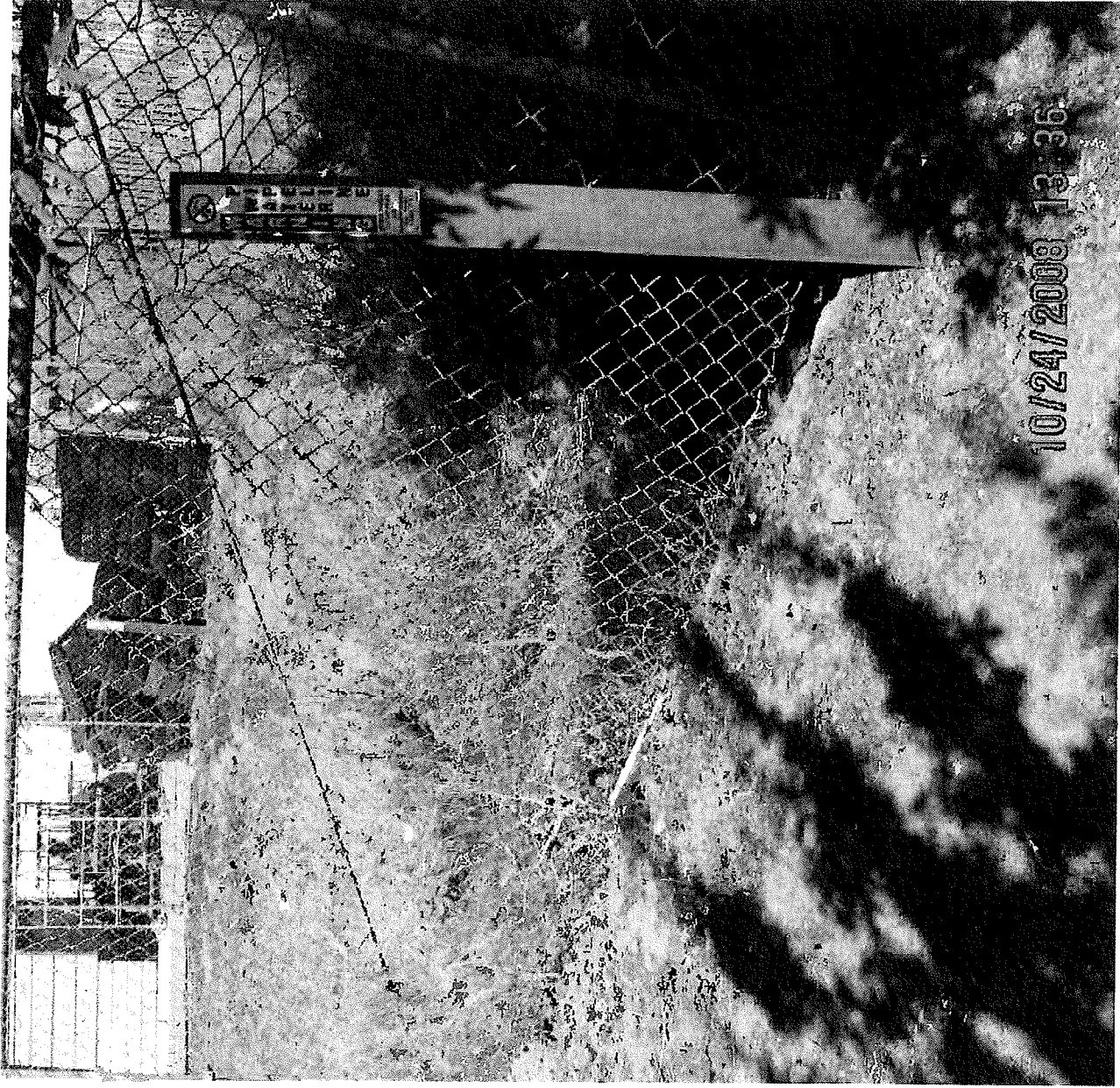
UV resistant plastic markers installed on 10/24/2008 identifying the location of an underground water main crossing under Rio Linda Creek
