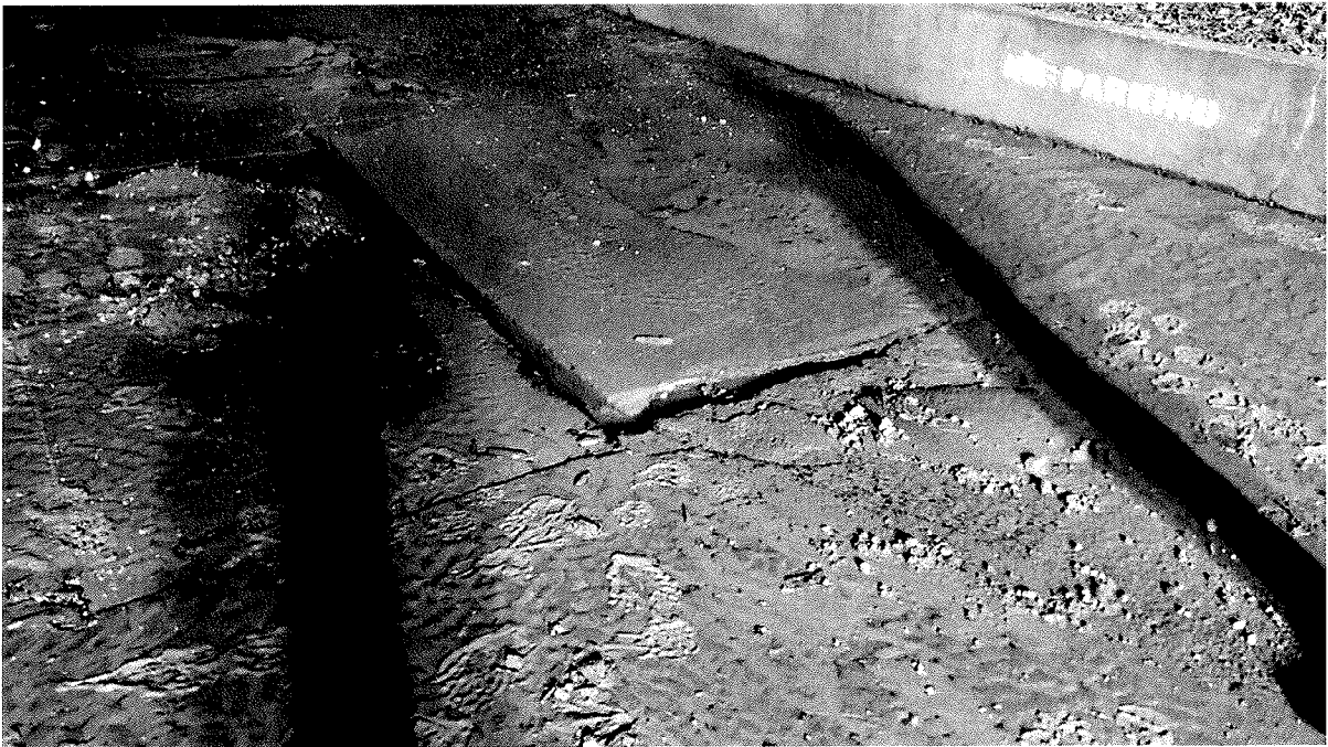
This photo shows the damage to the asphalt in the condominium complex parking area caused by the water main failure.
