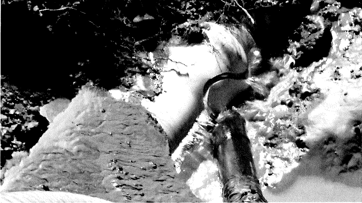
This photo shows the cracked and split bell end of the failed section of C-900 water main.
