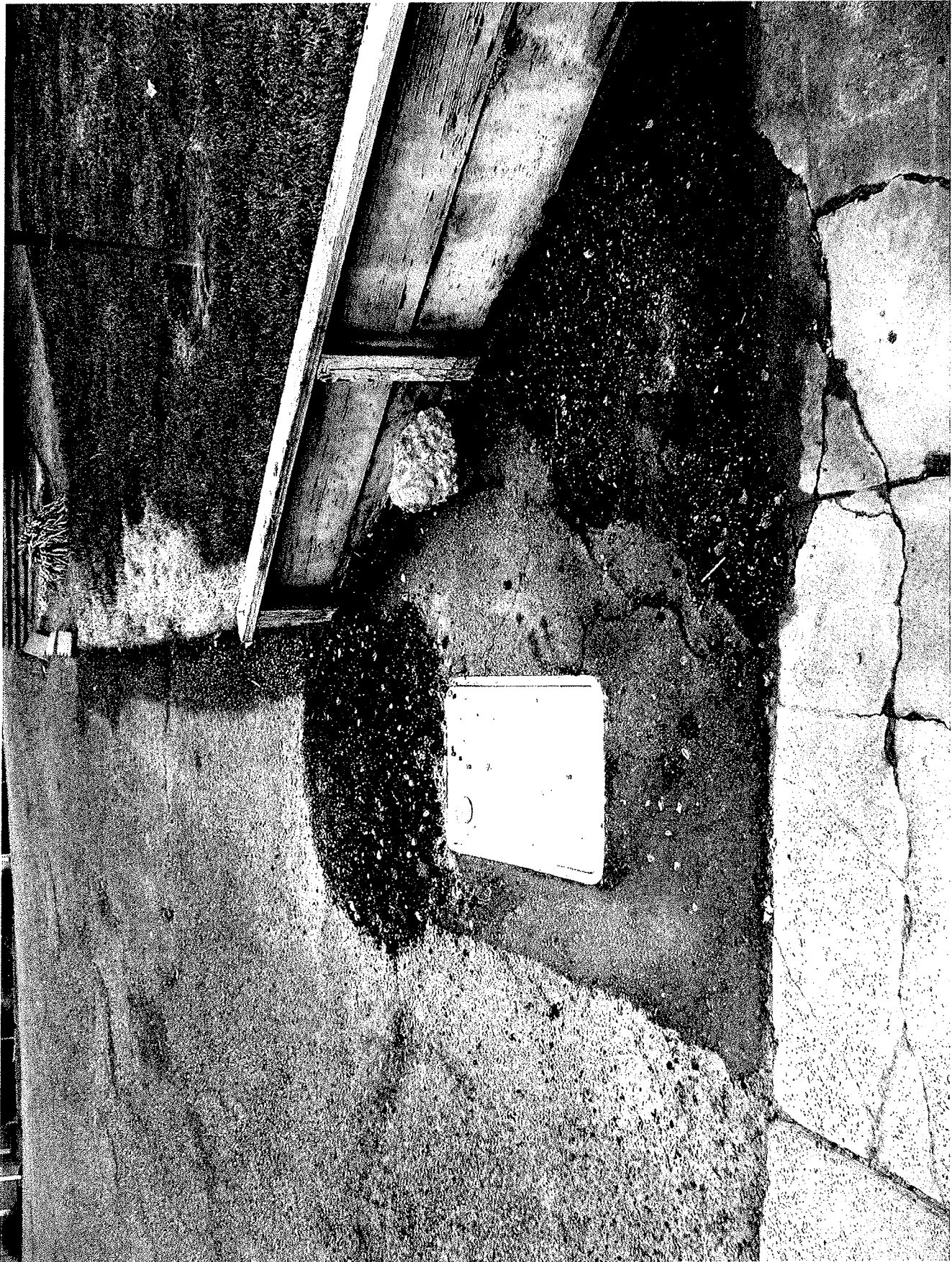
3305 EDISON AVE — LOOKING @ METER
