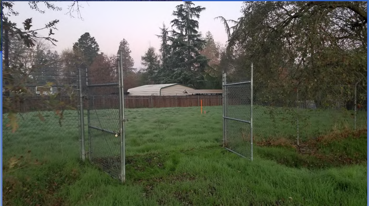
Well 78 – Butano/Cottage Production Well and Pumping Station Site
