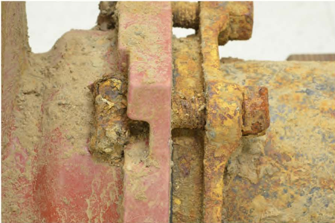
(a) Valve 1 coupling bolt 1A
