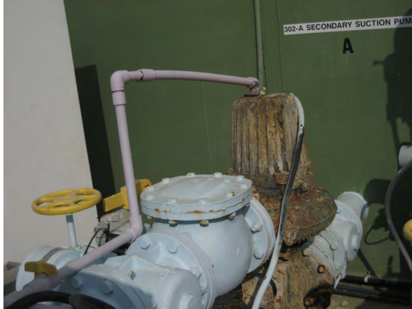
Figure 4. Score = 4: Poor Condition
