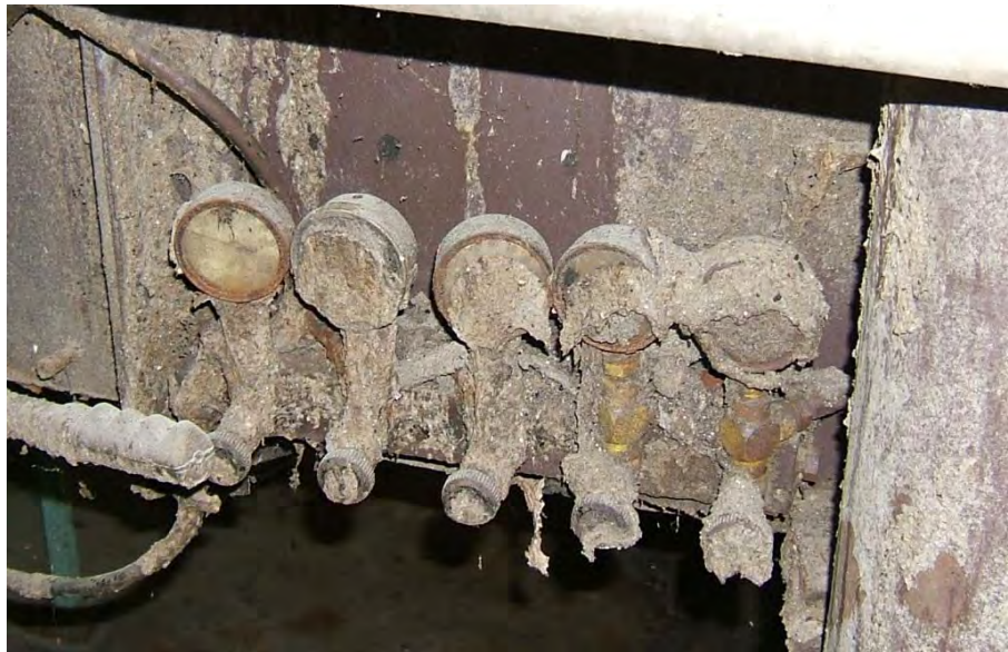
Figure 6. Score = 5: Failed Condition Example 2
