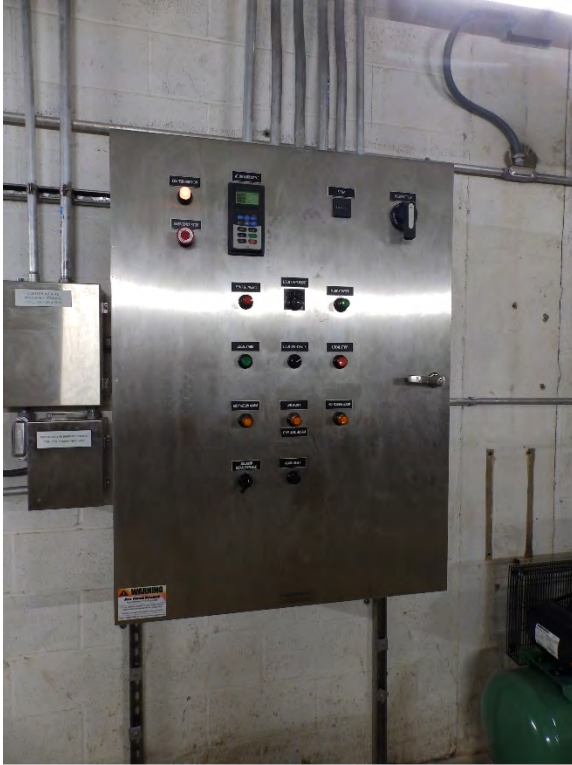
Electrical Equipment in Excellent Condition: Score = 1
