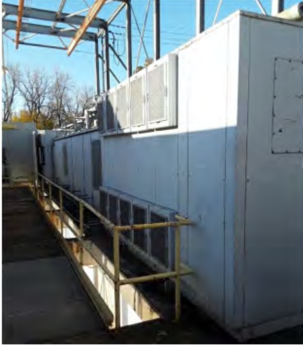
Electrical Equipment in Fair Condition: Score = 2
