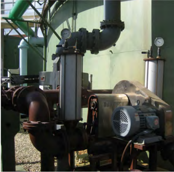
Mechanical Equipment in Fair Condition: Score = 2
