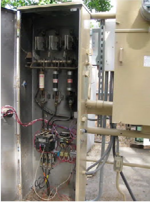
Electrical Equipment in Poor Condition: Score = 4
