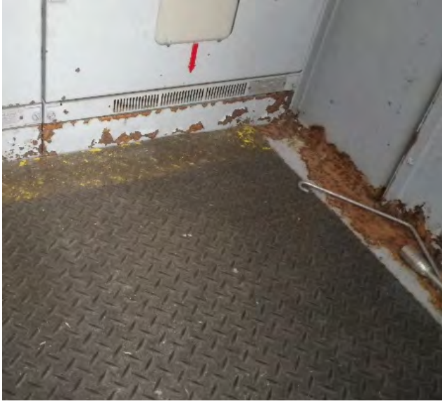
Electrical Equipment in Moderate Condition: Score = 3
