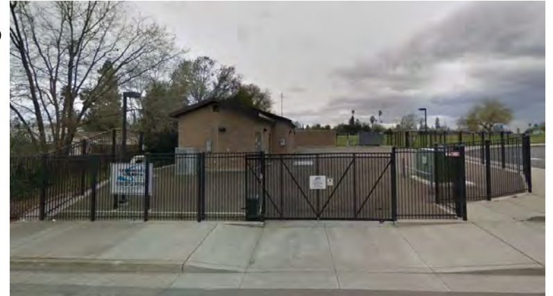
Asset: Well & Pump Station (Well N38 Coyle)
