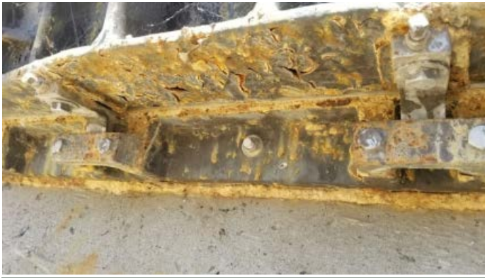
Structural Asset in Poor Condition: Score = 4
