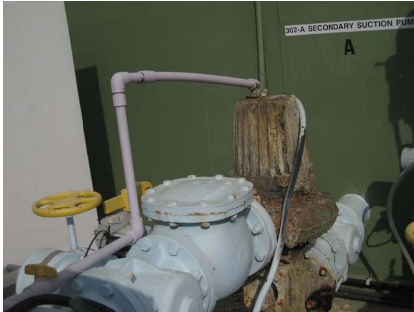
Figure 4. Score = 4: Poor Condition
