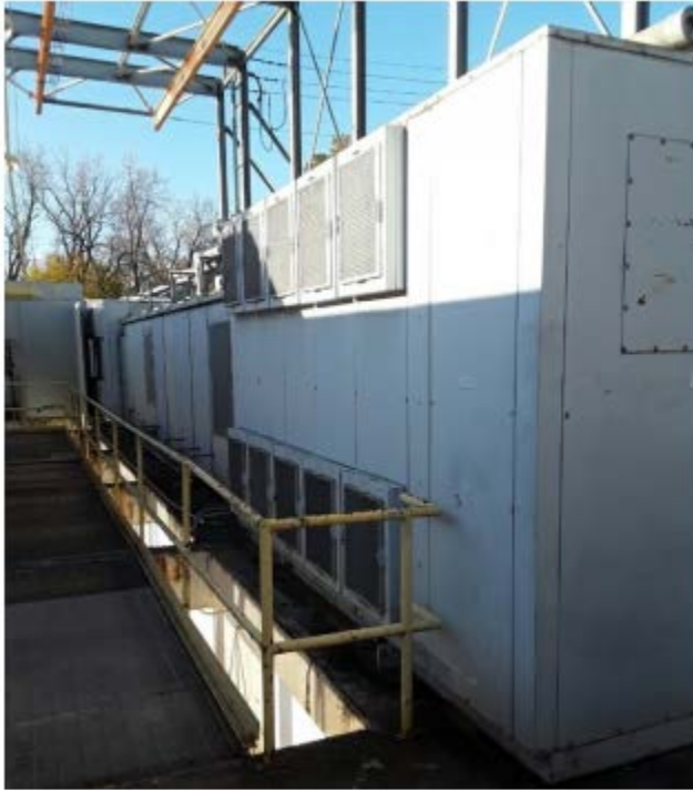
Electrical Equipment in Fair Condition: Score = 2
