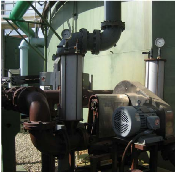
Mechanical Equipment in Fair Condition: Score = 2
