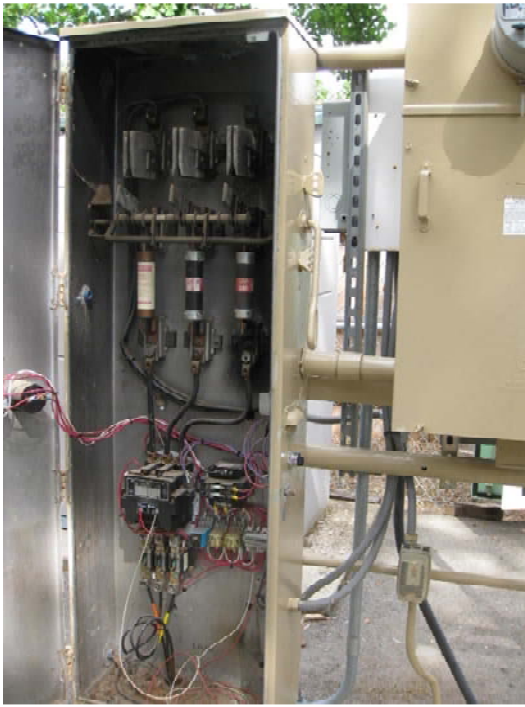
Electrical Equipment in Poor Condition: Score = 4
