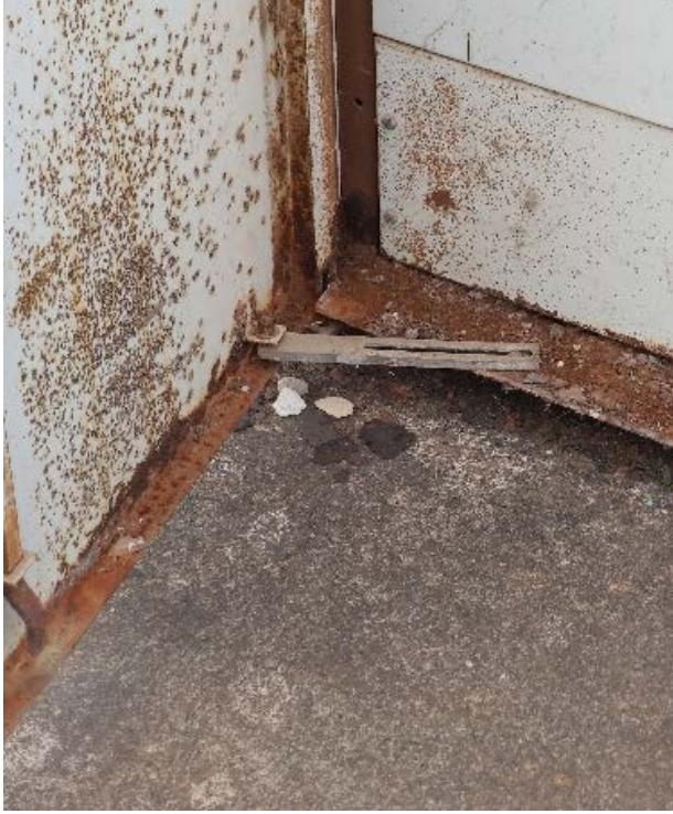
Electrical Equipment in Failed Condition: Score = 5
