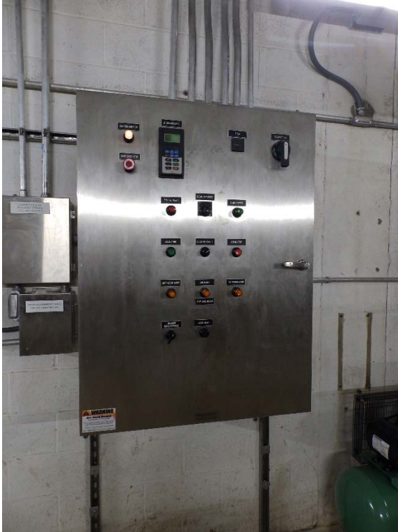
Electrical Equipment in Excellent Condition: Score = 1
