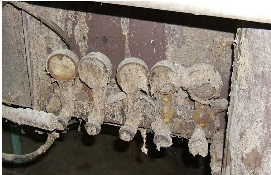
Figure 6. Score = 5: Failed Condition Example 2
