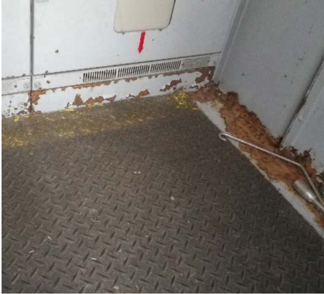
Electrical Equipment in Moderate Condition: Score = 3
