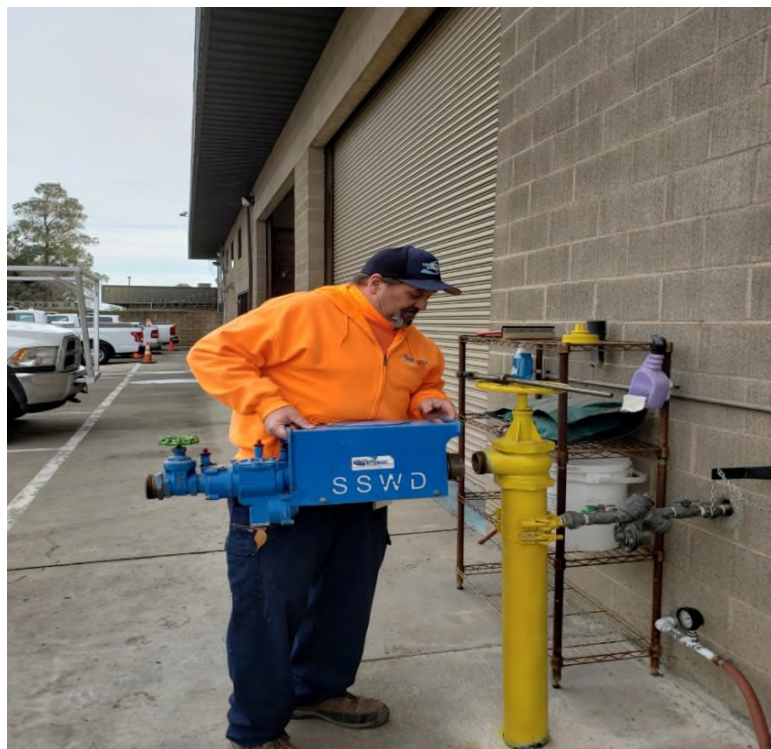
Previous Backflow Testing Setup
